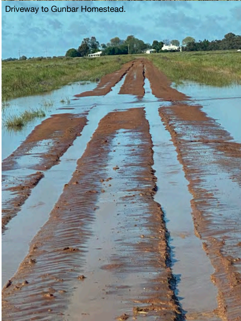
Water running under the culvert near cattle yards.
